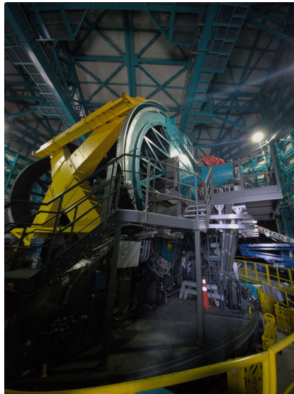
wide angle view of the telescope mount assembly (TMA). The large yellow "X" structure is there for construction purposes and will be removed to accommodate the M1M3 mirror cell in operation
